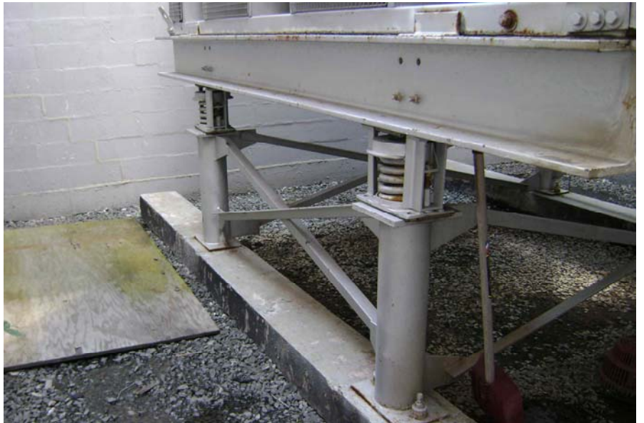
Figure S2: Existing cooling tower support framing. Note unbolted spring isolators.
