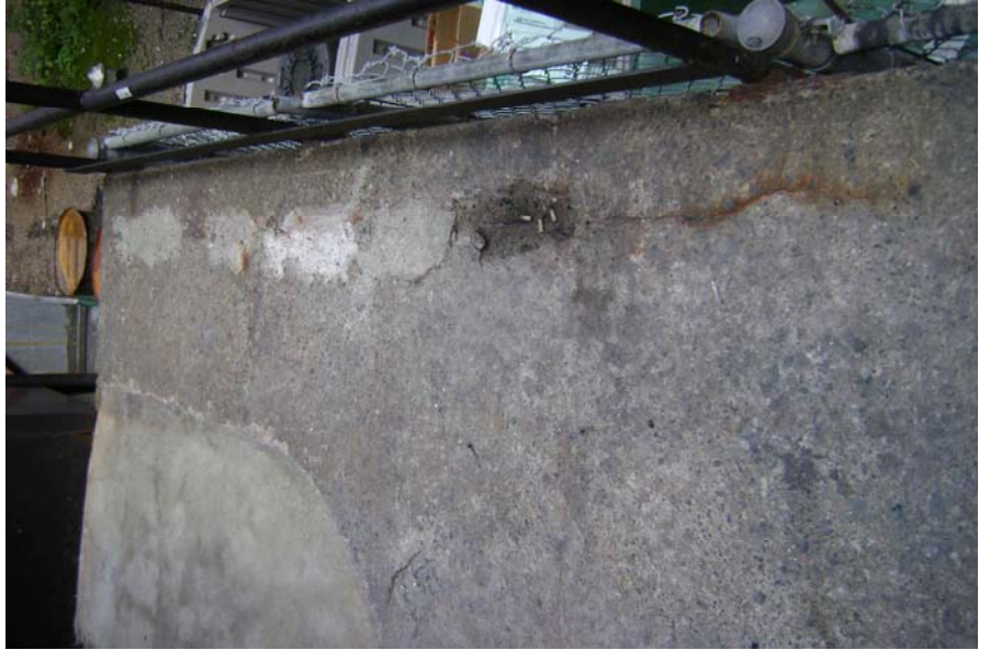
Figure S4: Spalled concrete at the Granville Street cantilevered slab.
