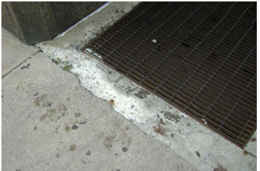
Figure S3: Spalled concrete at transformer grating in Granville Street ramp slab.
