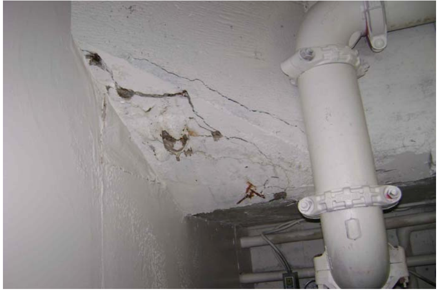
Figure S6: Cracked, spalled concrete at the soffit of the main entrance stair slab, Hollis Street level.
