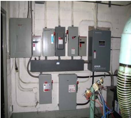
Photo 1.2; Automatic transfer switch on far right.
