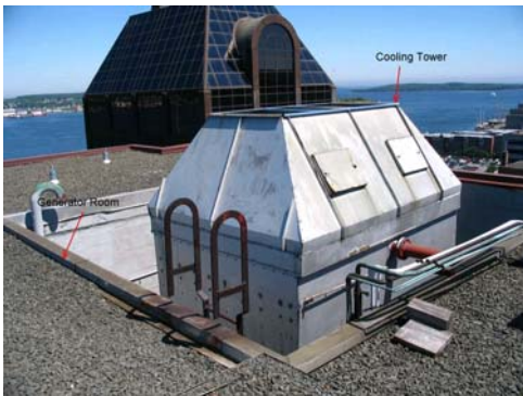
Photo 1.4; Shows the generator room location and cooling tower
