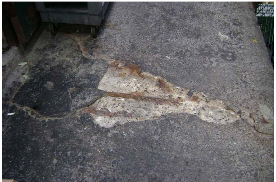
Figure S5: Spalled concrete and corroded reinforcing steel at the Granville Street cantilevered slab.
