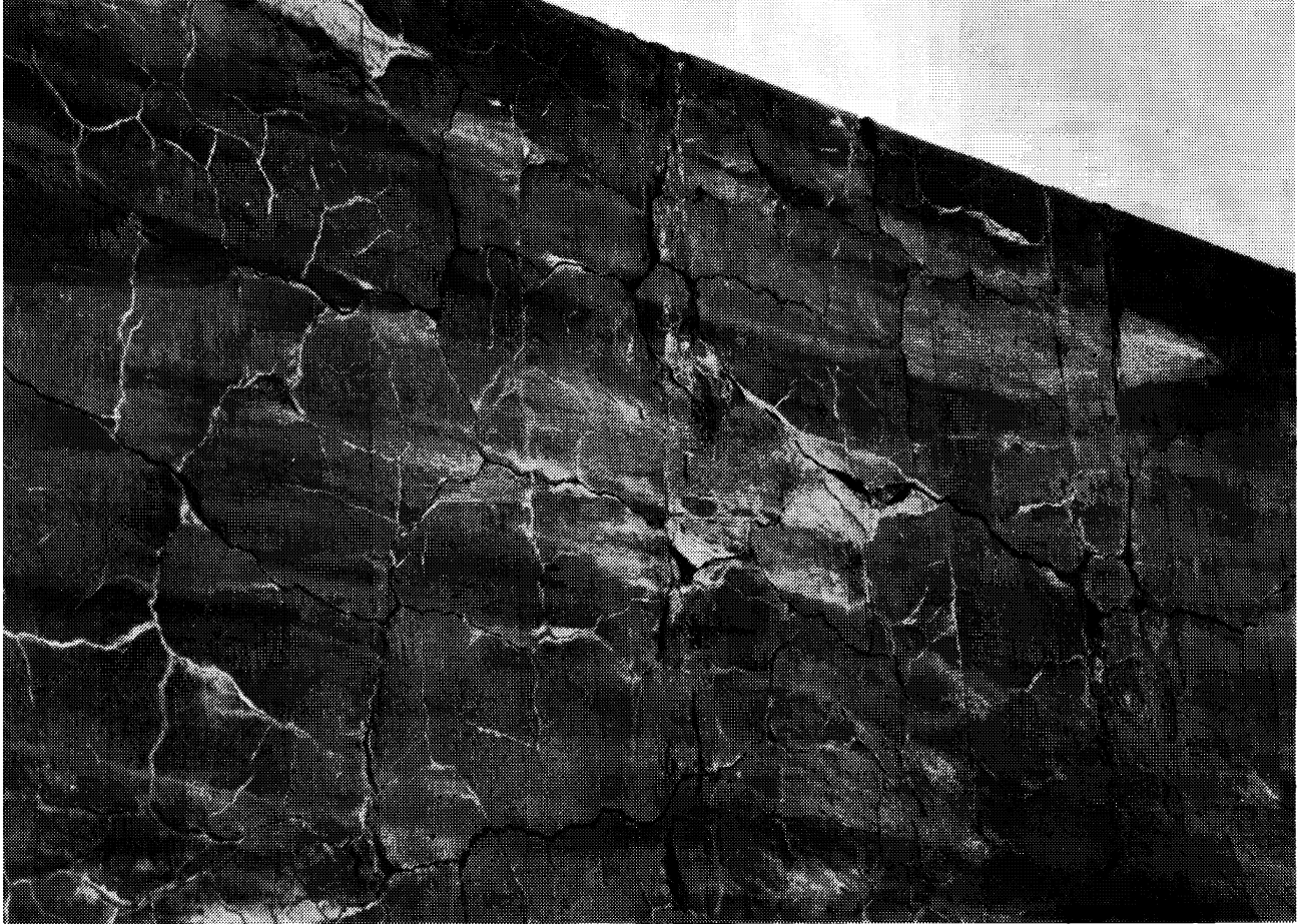
Figure 13. Example of a concrete structure in the advanced stages of alkali-aggregate reactivity. Once the reaction has begun, deterioration of the structure is accelerated by freeze-thaw cycles.
