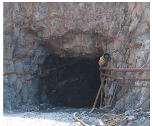
Photograph of the entrance to Azure Resources Corp.'s decline at the Mooseland gold deposit in Halifax County. The decline was started in the summer of 2003, and work continues to access target zones where an underground bulk sample will be collected by the company.
