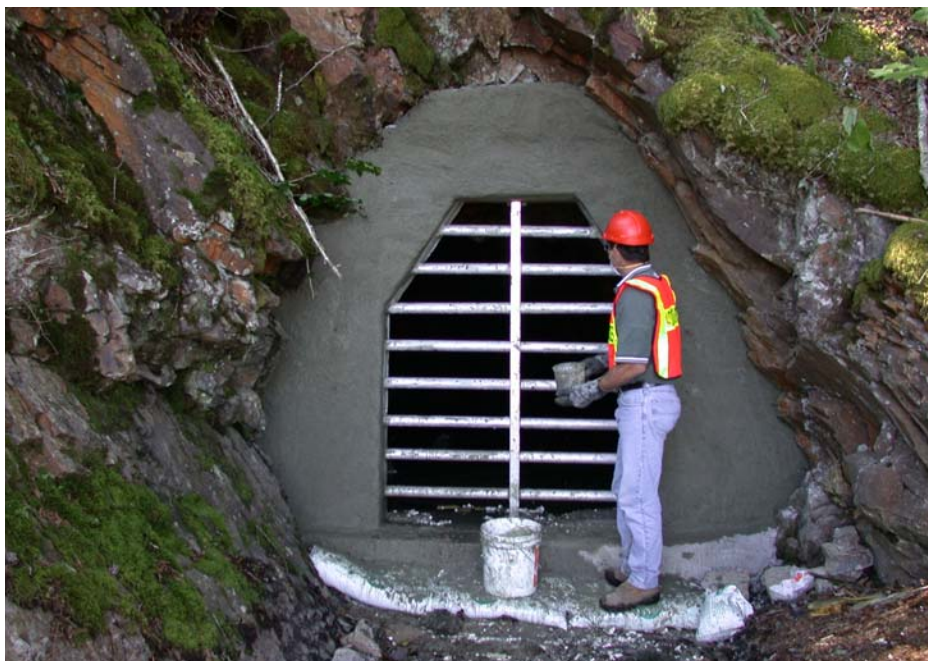
Regional Geologist Don Weir works to remediate a mine opening at Lake Charlotte.
