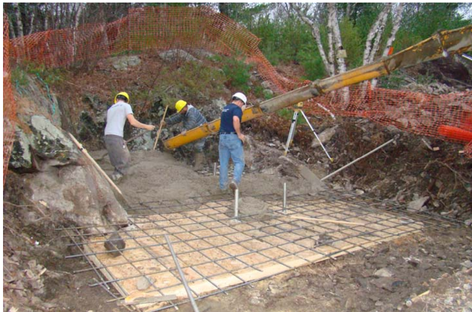
Concrete cap on the King Fissure shaft in North Brookfield, Queens County.
