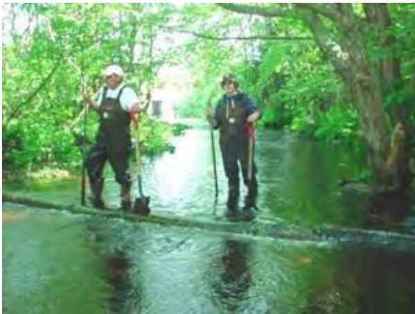
The Salmon River Salmon Association crew members finish a digger log installation on Belliveau Brook, Digby Co.
