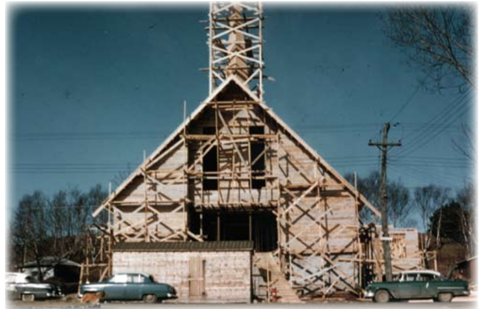
These photos show the construction of Stairs church on Hester Street, beginning with the empty lot (top left), completion of the framing in above and the new spiritual home opening its doors to the congregation in 1959.
