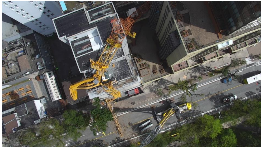
Photo 1: Aerial View of 1400 block of South Park Street Halifax after the collapse. Credit: Halifax Regional Fire & Emergency
