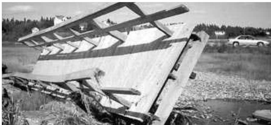
Juan's destruction to walkways at Conrad's Beach
