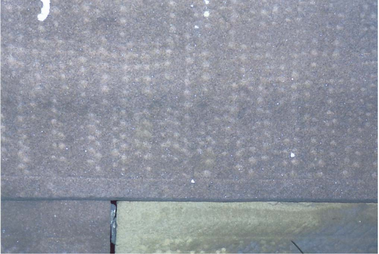
Figure 2. This photograph illustrates the condition of sandstone blocks found in the foundation of the Judique Manse. Note how the chisel marks (round spots) made when the stone was cut over a century ago are still evident.
