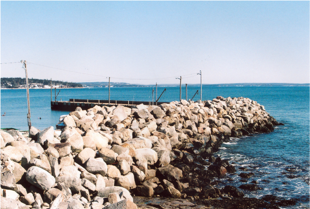
Figure 5. Examples of common breakwater construction methods; large armour stone breakwater protecting an older creosote-framed, interlocking bay and stone ballast breakwater located at Fox Point, St. Margarets Bay.
