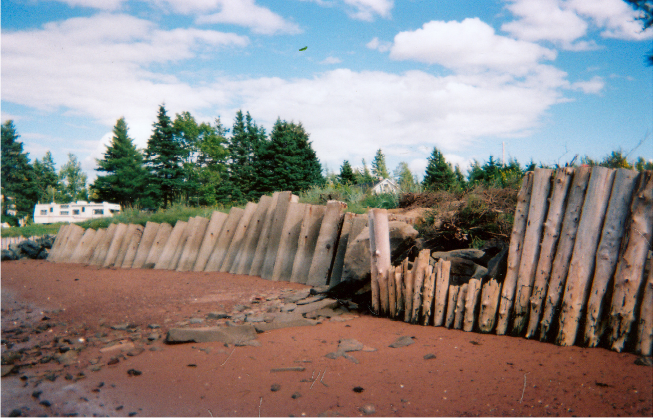
Figure 3. Retaining wall constructed from concrete 'L shaped' forms located west of the Ship Rail Provincial Park.
