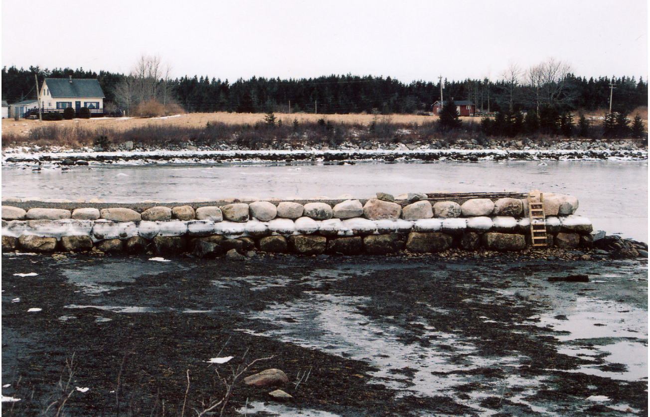
Figure 15. A well constructed and durable stone pier built using oval shaped granite boulders, Blandford, Mahone Bay. Note the row over row staggered placement of stone.
