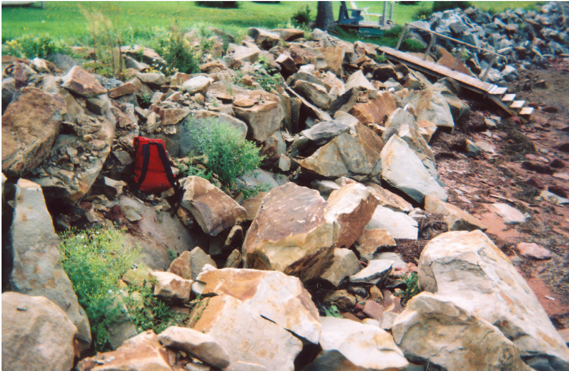
Figure 10. Collapsed retaining wall showing fragmented boulders, substandard sandstone armour stone, improper placement of stone on an eroding till substrate, failure to anchor the toe of the wall below the actively eroding shoreface, and improper use of geotextile.
