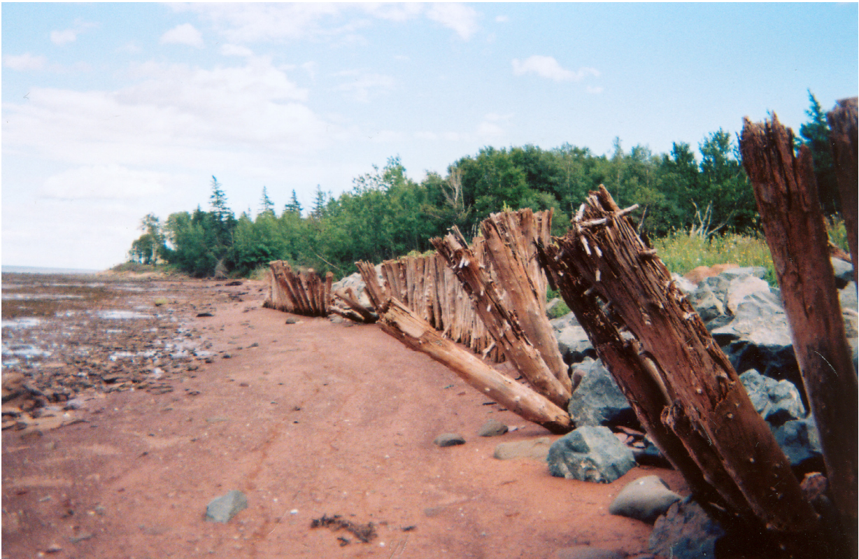
Figure 6. View of a failed wood retaining wall later partially backfilled with armour stone. Note the lack of horizontal bracing.
