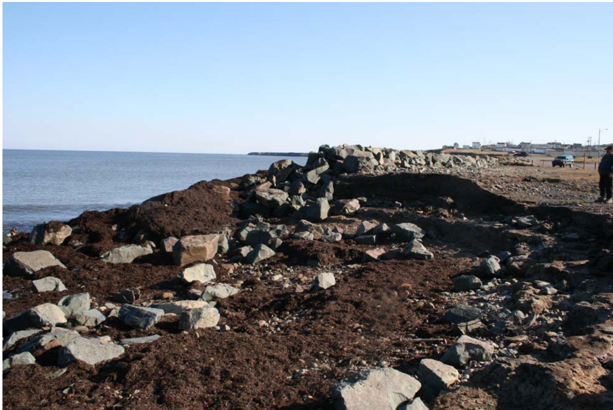
Figure 6. Boulders strewn near the low-tide level of the beach is evidence of erosion of the north end of the abutment at Dominion Beach.
