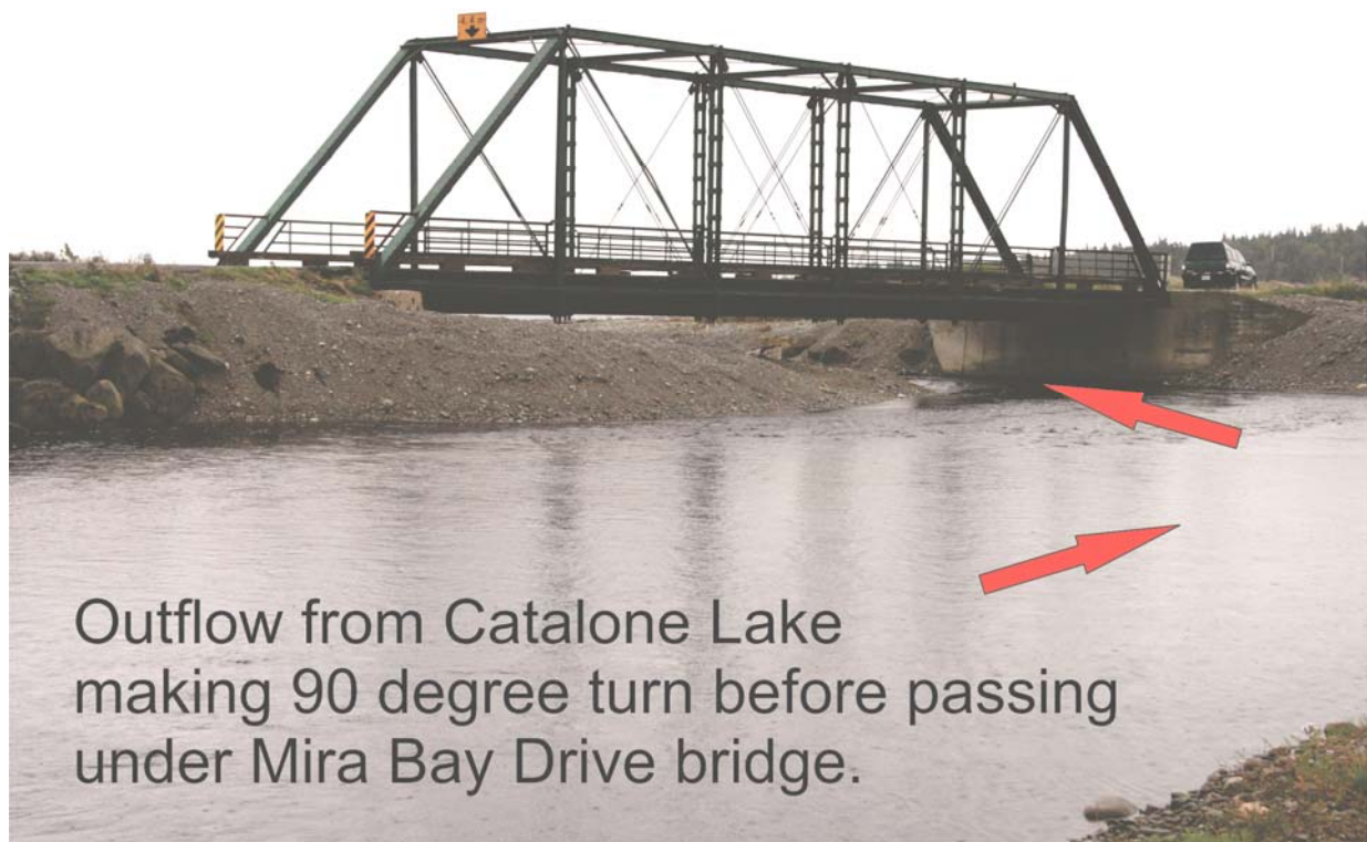
Figure 7. Photograph illustrating the wide, shallow, meandering nature of the drainage channel on the landward side of Mira Bay Drive Bridge.
