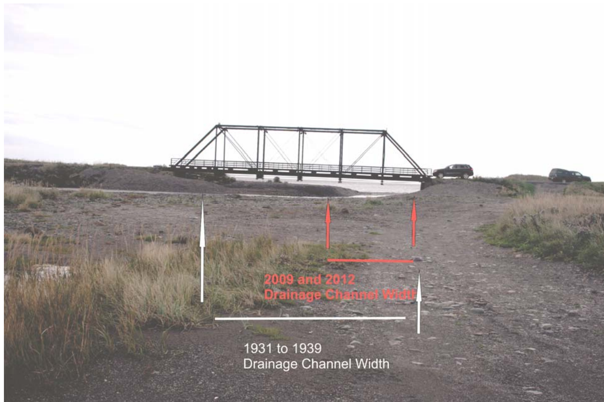
Figure 5. Photograph showing the narrow drainage channel under Mira Bay Drive Bridge, looking seaward from the flood-tide dominated bar.
