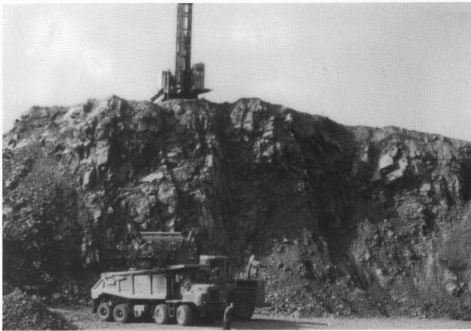
Figure 23. The aggregate quarry at Folly Lake, Colchester County, is owned by Permanent Lafarge, Division of Lafarge Canada Inc. The operation is active on demand.
