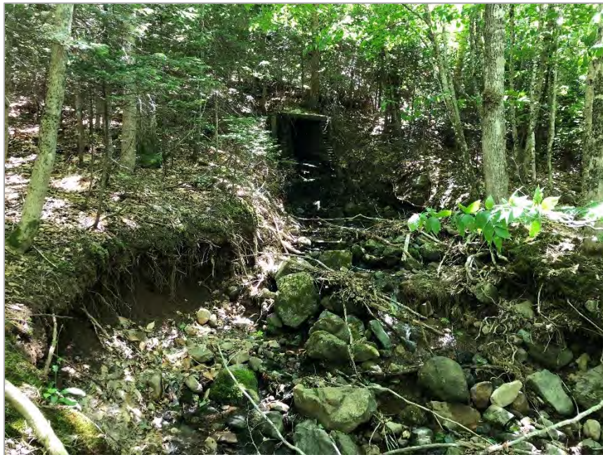
Figure 5. Downstream end of culvert below Westchester Road; a hanging culvert along unnamed stream 2, situated approximately 1.5 m above the streambed creating a barrier to fish. July 13, 2022.
