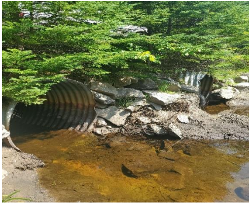
Photo 32. Evidence of alteration along WC20.
