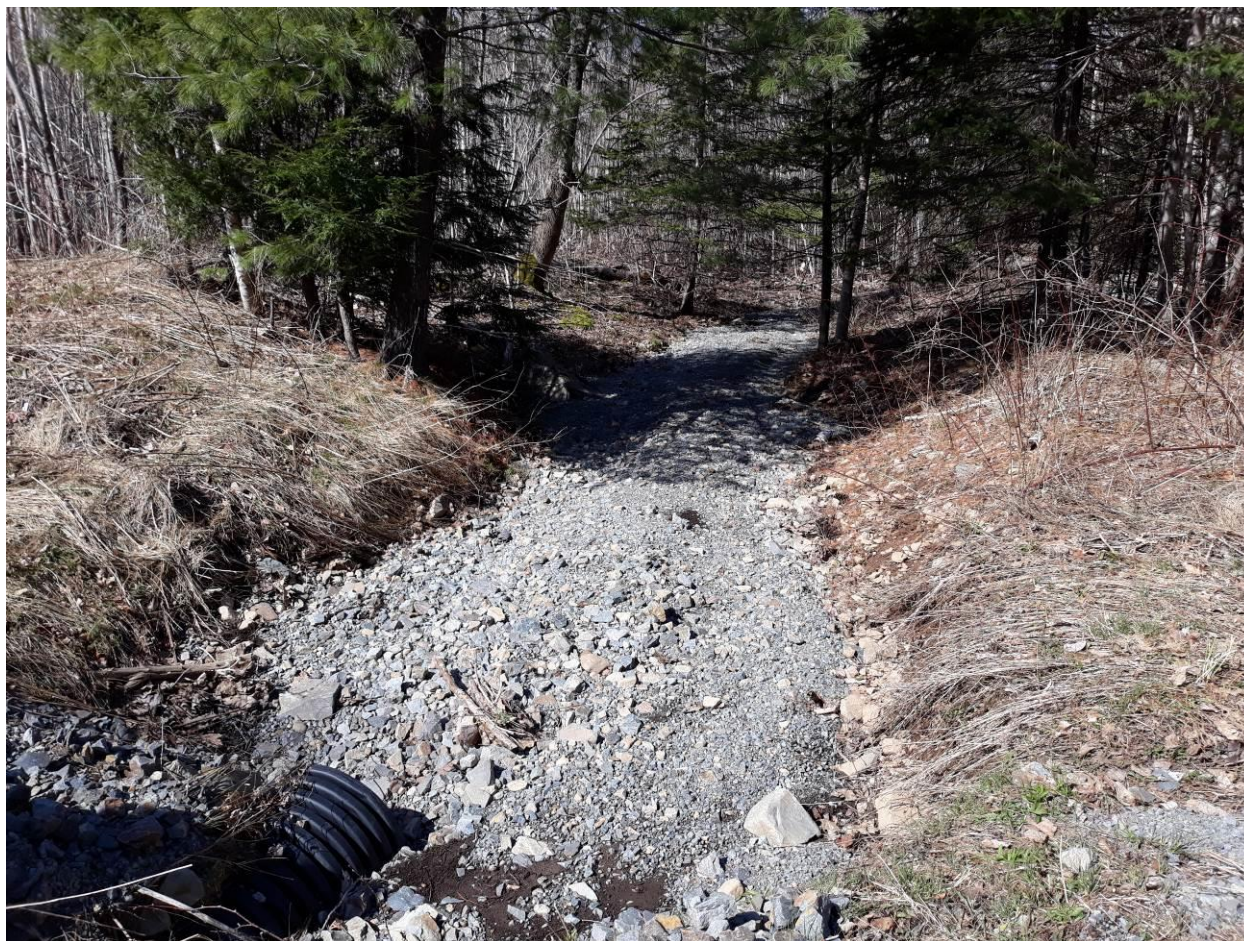
Figure 7. Downstream end of culvert on the unnamed stream where it passes beneath the quarry road. Photo by S. Timpa, April 10, 2024.
