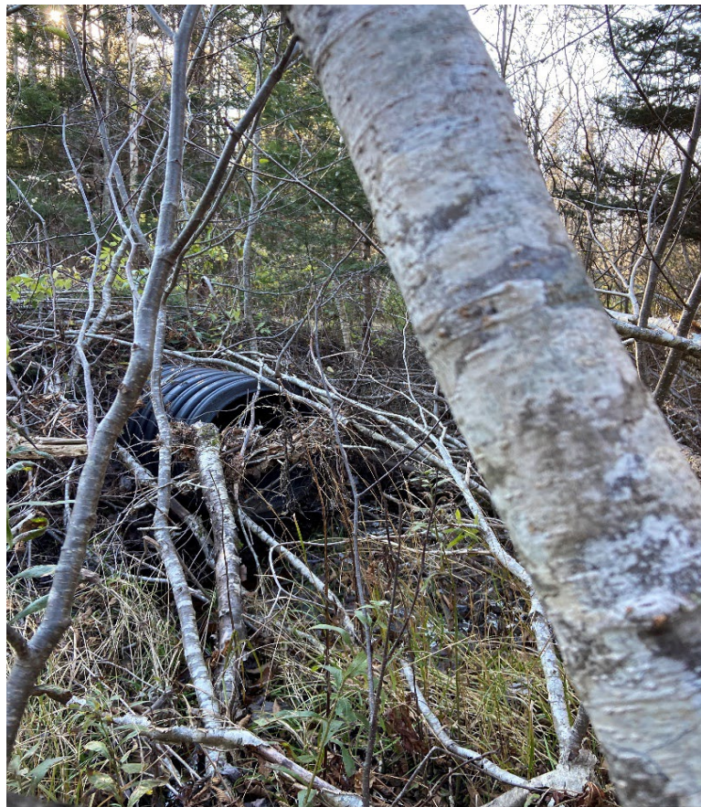
Photo 3: Feature 1 (Perched, partially blocked culvert, upstream of crossing)
