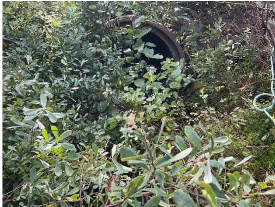
Photo 3: Evidence of alteration along WC2.
