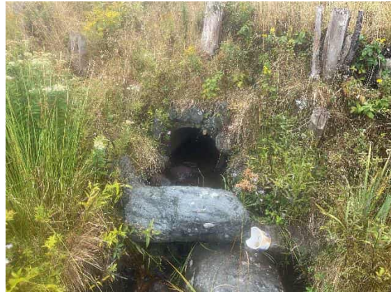
Photo 16: Evidence of alteration along WC13.
