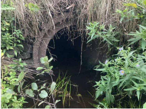
Photo 13: Evidence of alteration along WC11.
