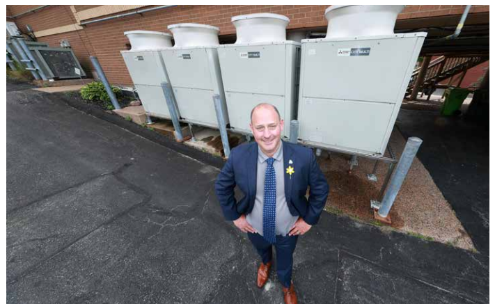
New heat pumps at the Canadian Cancer Society's The Lodge That Gives were made possible with funding from the Sustainable Communities Challenge Fund.
