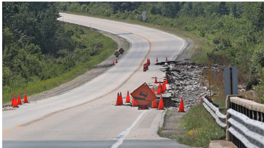
Hwy 103 Rain Damage
