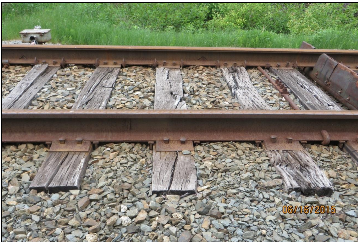
M.P. 42.8 - HOT BOX AND DRAGGING EQUIPMENT DETECTOR New wood ties required to hold track gauge across the detector
