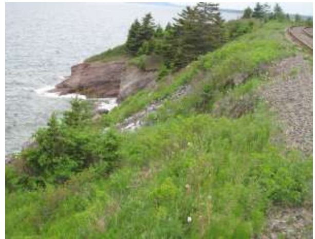
Photo 32 – Mile 55.1: Subsidized Line Sloughing Near West End of Slope
