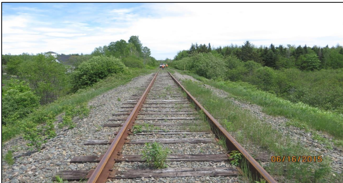
M.P. 33.37 – Tangent Track Vegetation in roadbed – Defect ratio for ties at 45% - 55%
