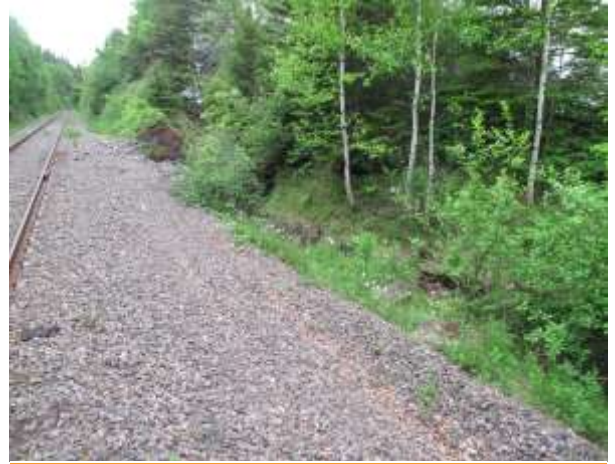
Photo 42 – Mile 68.3: Subsidized Line Significant Slope Movement
