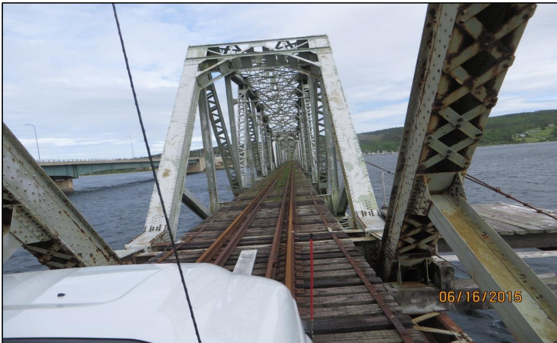
M.P. 57.7 – BRIDGE - GRAND NARROWS Swing Span at east end of bridge Manual interlocking between M.P. 57.4 and M.P. 57.9
