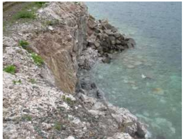
Photo 28 – Mile 54.6: Subsidized Line Local Sloughing Near Crest of Cliff June 18, 2014
