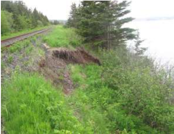
Photo 37 – Mile 60.1: Subsidized Line Vertical Displacement at Crest of Slope June 18, 2014
