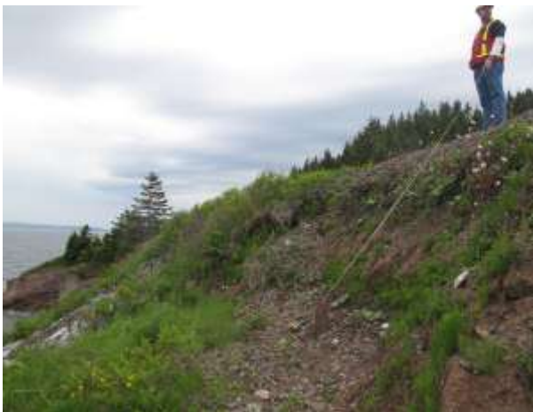
Photo 33 – Mile 55.1: Subsidized Line Vertical Displacement at Crest of Slope
