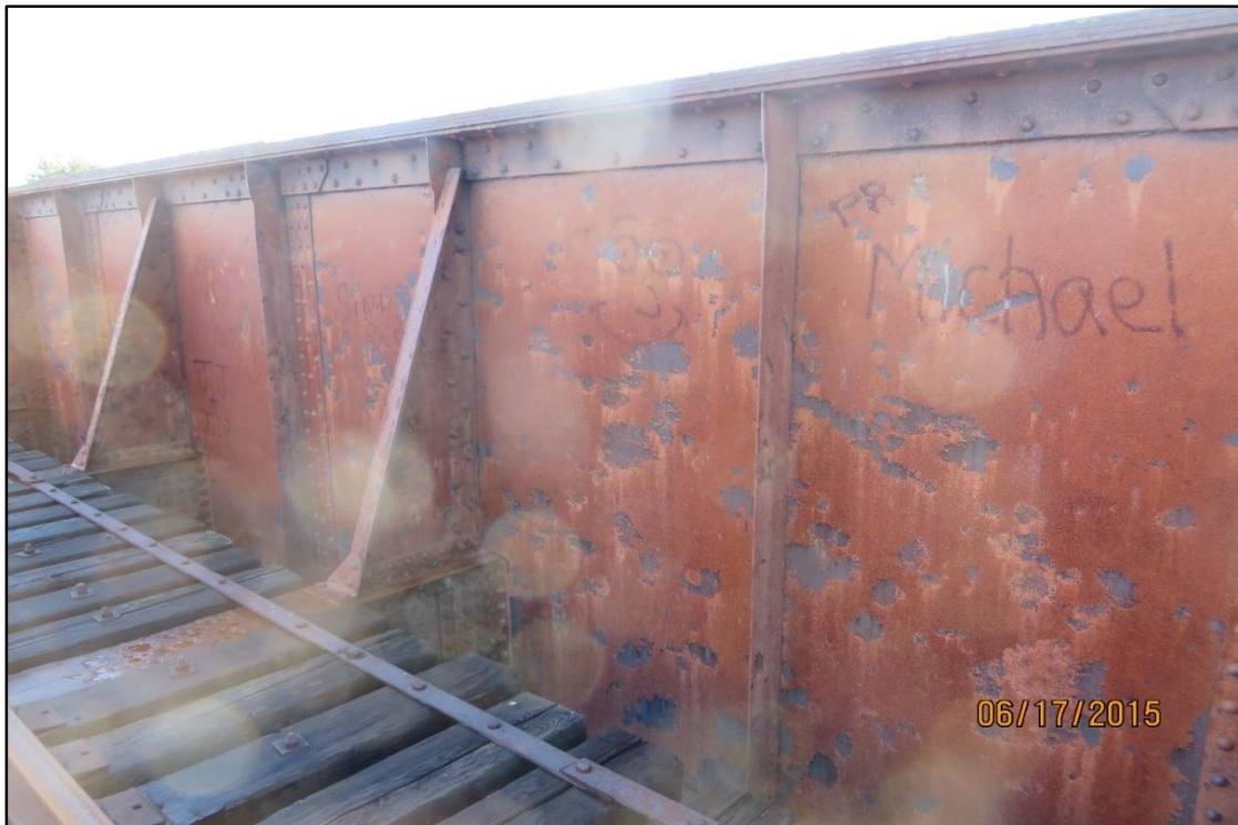
M.P. 103.3 – BRIDGE PLATE Heavy rust
