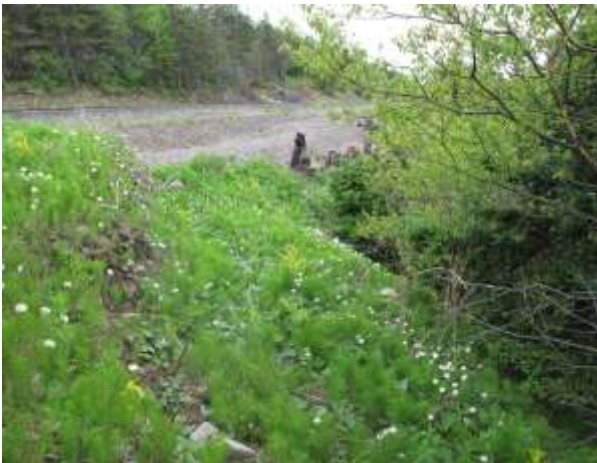
Photo 14 – Mile 3.0: Non Subsidized Line Crest of Slope (East Side): Sloughing June 18, 2014
