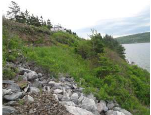
Photo 34 – Mile 55.1: Subsidized Line Vertical Displacement at Crest of Slope
