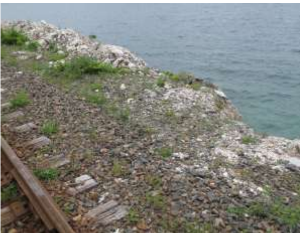
Photo 27 – Mile 54.6: Subsidized Line Area Between Line and Cliff June 18, 2014
