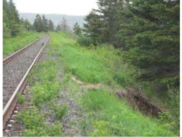
Photo 36 – Mile 60.1: Subsidized Line North Side of Line: Sloughing at Crest June 18, 2014
