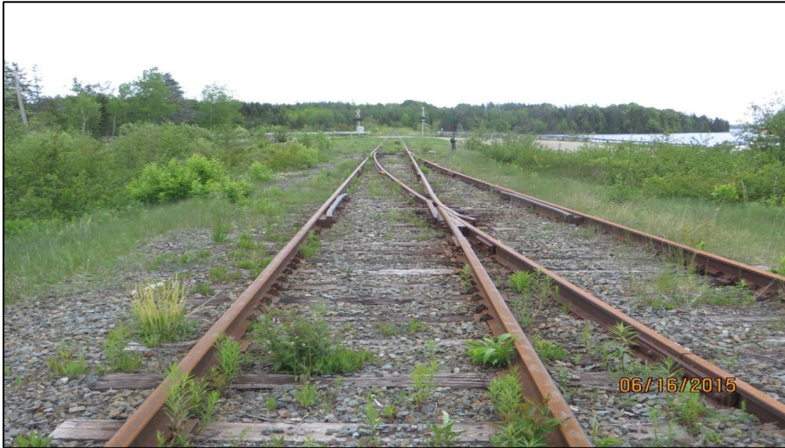
M.P. 41.3 – East Turnout - ORANGEDALE No. 10 Turnout with Spring Frog
