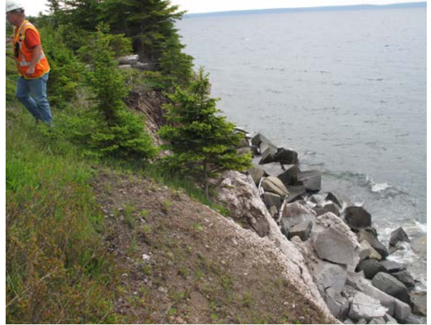
Photo #54 - Mile 53.8: Subsidized Line Local Sloughing Near Crest
