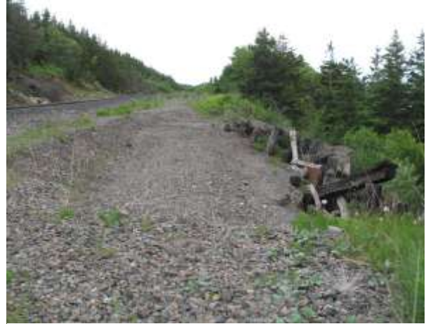
Photo 13 – Mile 3.0: Non Subsidized Line Crest of Slope/Top of Existing Retaining Wall June 18, 2014
