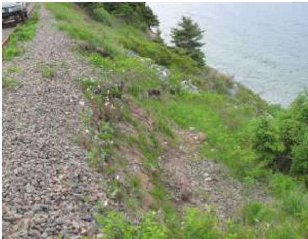
Photo 31 – Mile 55.1: Subsidized Line Sloughing Near East End of Slope
