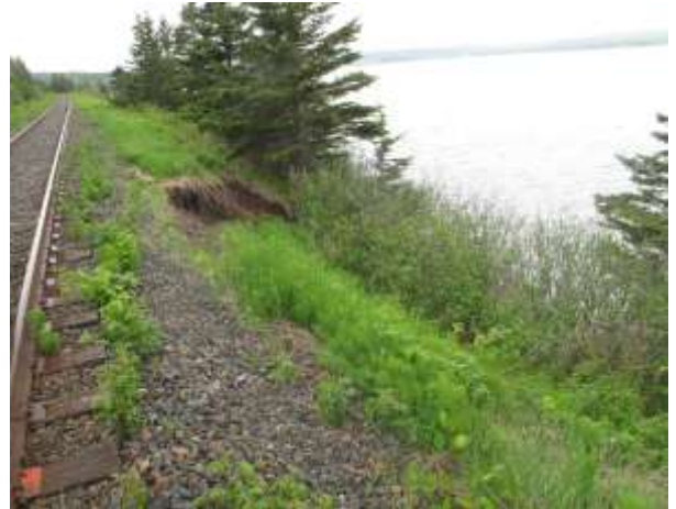
Photo 38 – Mile 60.1: Subsidized Line Vertical Displacement at Crest of Slope June 18, 2014
