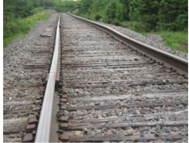
Photo 8 – Mile 2.9: Non Subsidized Line Line Settlements June 18, 2014
