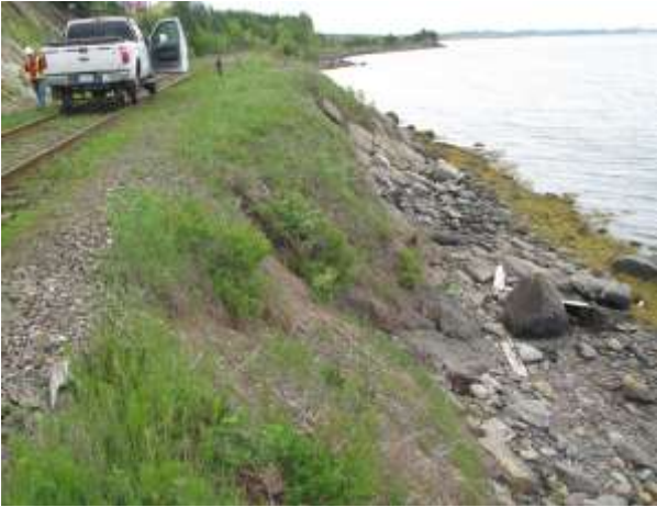
Photo 18 – Mile 8.5: Non Subsidized Line Westerly Looking Easterly: Sloughing
