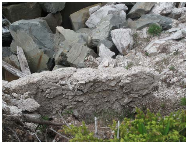
Photo #58 - Mile 53.8: Subsidized Line Soughed Material at Toe
