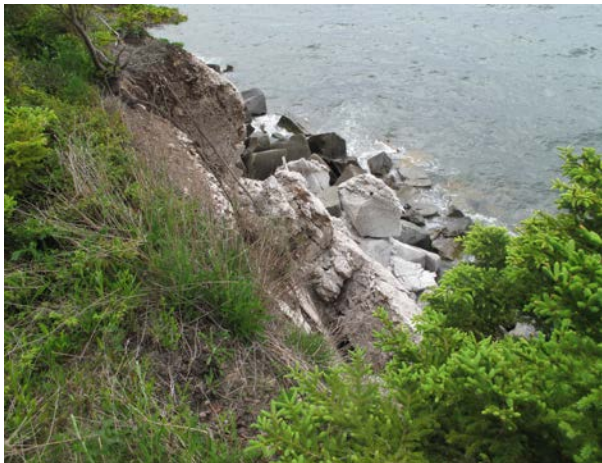
Photo #55 - Mile 53.8: Subsidized Line Toe of Embankment
