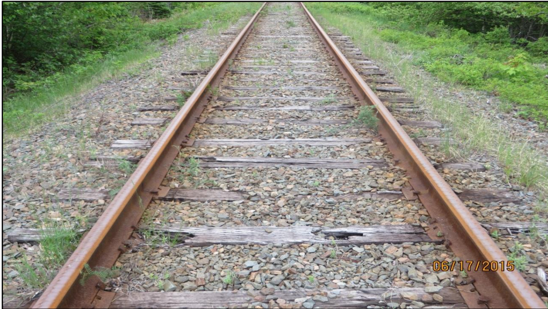
M.P. 85.85 – TANGENT TRACK Tie Defect Ratio at 50% - 55%
