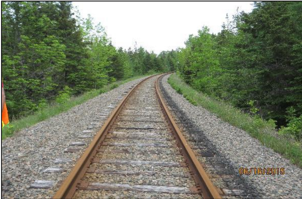
PHOTO M.P. 25.46 – Track alignment – R.H. Curve Good ballast cross-section and solid ties
