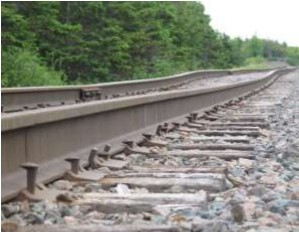
Photo 9 – Mile 2.9: Non Subsidized Line Side View Showing Line Settlements June 18, 2014
