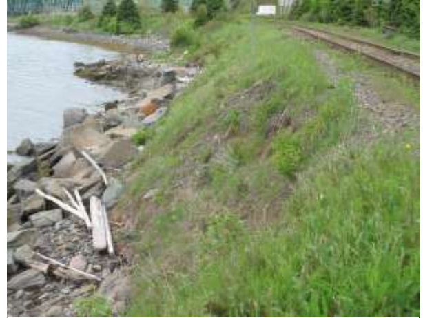
Photo 19 – Mile 8.5: Non Subsidized Line Easterly Looking Westerly: Sloughing
