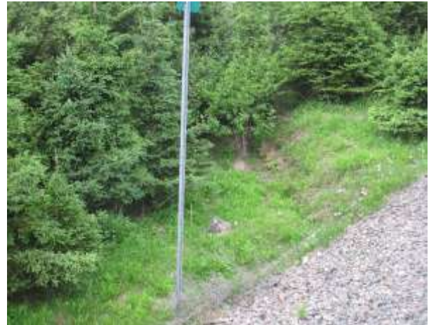
Photo 10 – Mile 2.9: Non Subsidized Line Crest of Slope: Sloughing June 18, 2014
