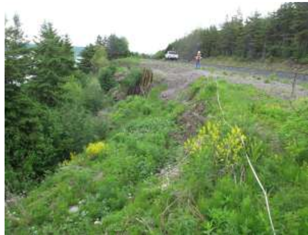
Photo 15 – Mile 3.0: Non Subsidized Line Crest of Slope (West Side): Sloughing June 18, 2014
