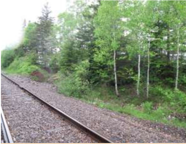
Photo 41 – Mile 68.3: Subsidized Line North Side of Line
