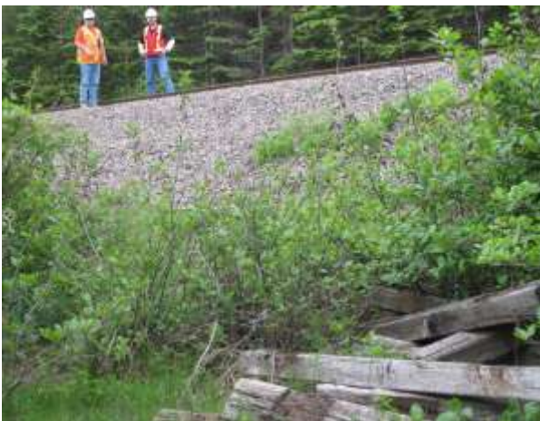
Photo 11 – Mile 2.9: Non Subsidized Line Toe of Slope: Bulging June 18, 2014
