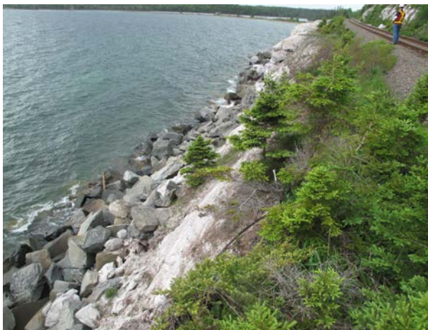
Photo #57 - Mile 53.8: Subsidized Line Toe of Embankment
