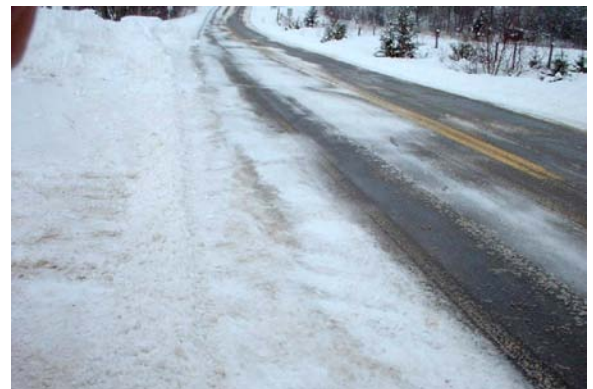
Road where anti-icing was not used.
